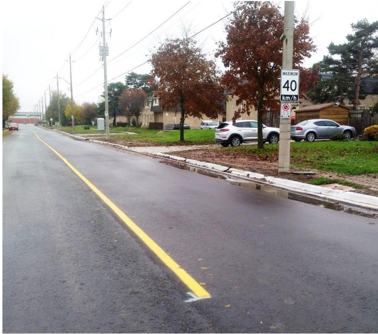
St. Vincent Street South facing South. Looking at recently paved Phase 1 before final restoration.
